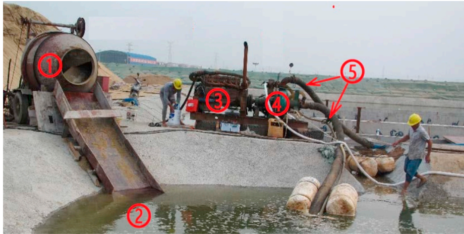
① Sand mixer ② Water-sand mixing tank ③ Pressure controller part ④ Sand pump ⑤ Water-sand conveyance part
